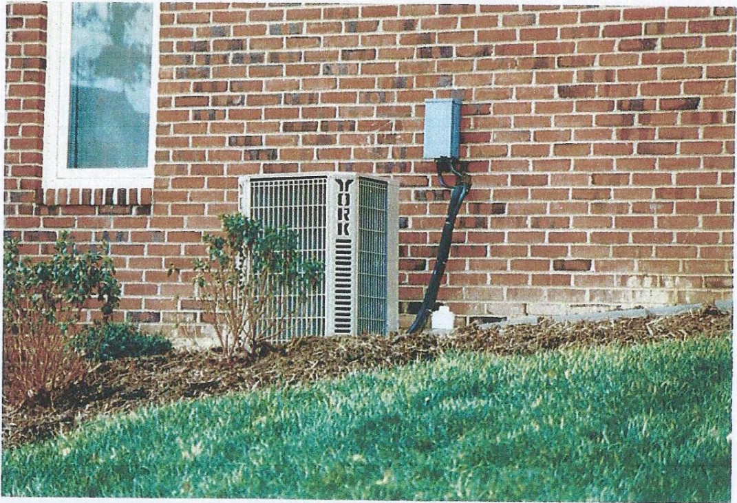
HVAC UNIT, Townhouse
